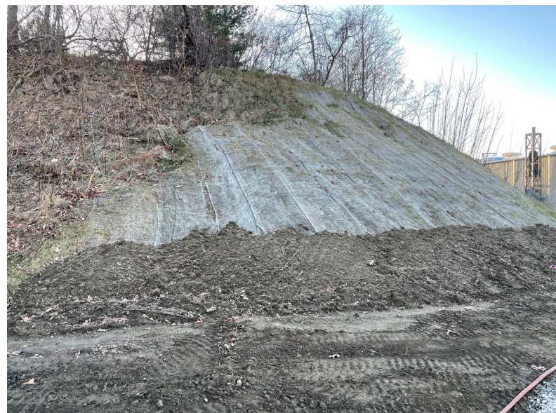
Figure 13 Bare soil on steep slope utilizing bio-degradable coconut fiber mat stabilization measures prior to vegetation growing in
