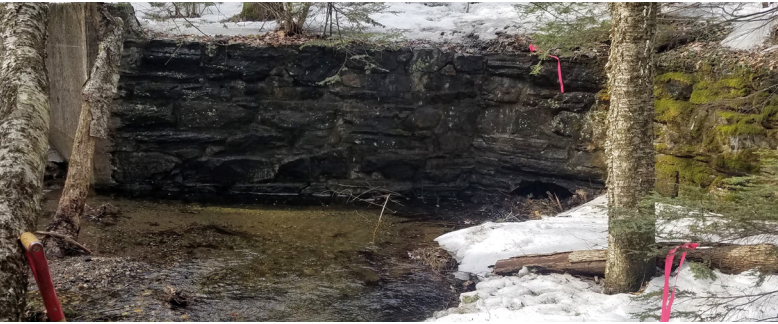
Figure 16 A partially-blocked culvert filled with sediment and debris.
