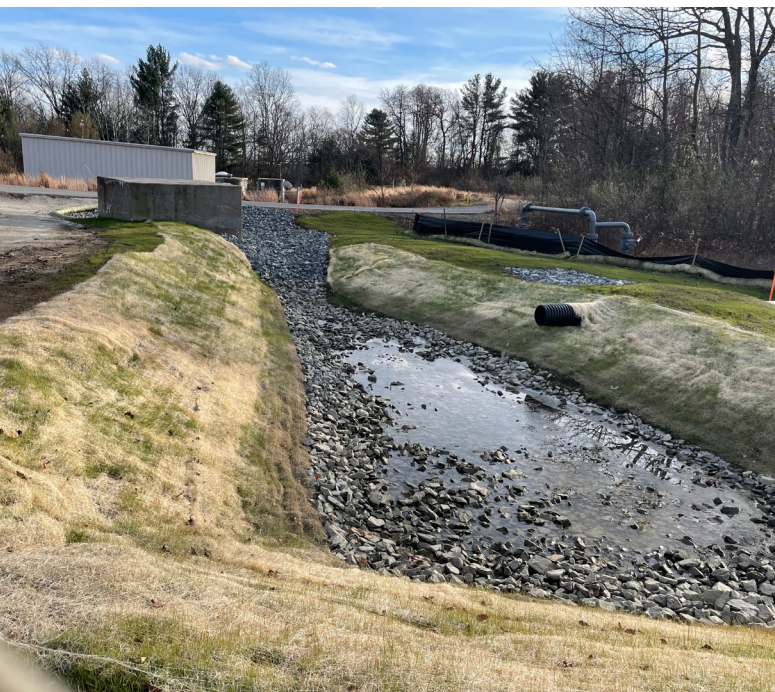
Figure 17 Stormwater detention basin that requires regular maintenance
