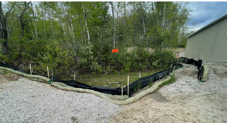
Figure 12 Siltation fencing and straw wattles installed to prevent mobilized sediments from entering a wetland
