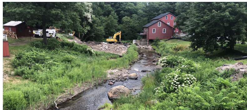
Figure 15 Dam removal and stream restoration in progress utilizing several bioengineering techniques including boulders, slope stabilization, and root wads.
