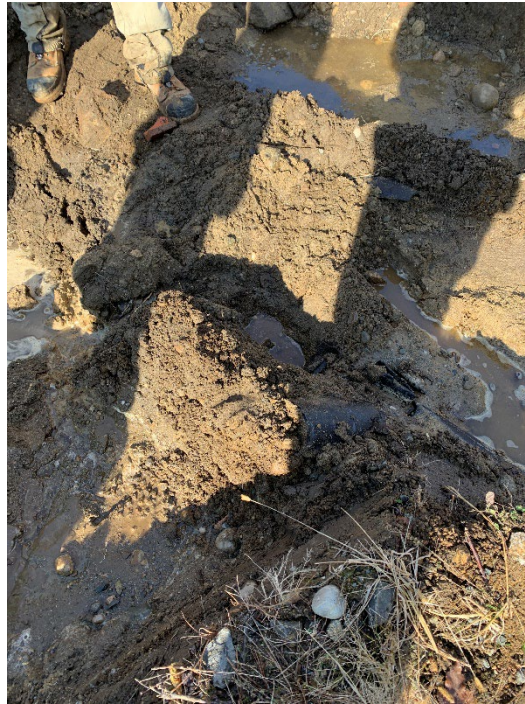
Photo 5 Beginning of drainpipe partially impacted by groundwater. Test pit 1.
