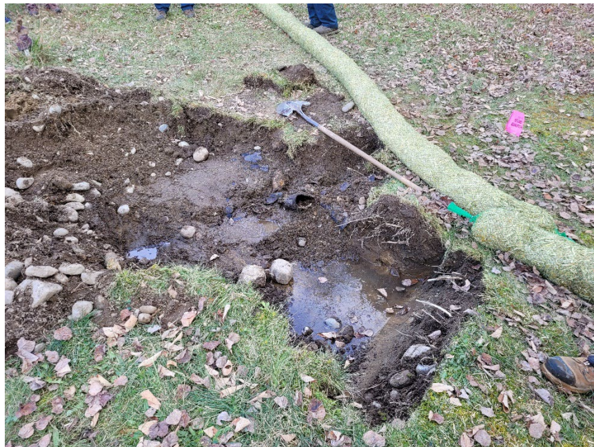
Photo 4 Drainpipe and eastern boundary of work area. Terminus of drainpipe underneath shovel. Test pit 2.
