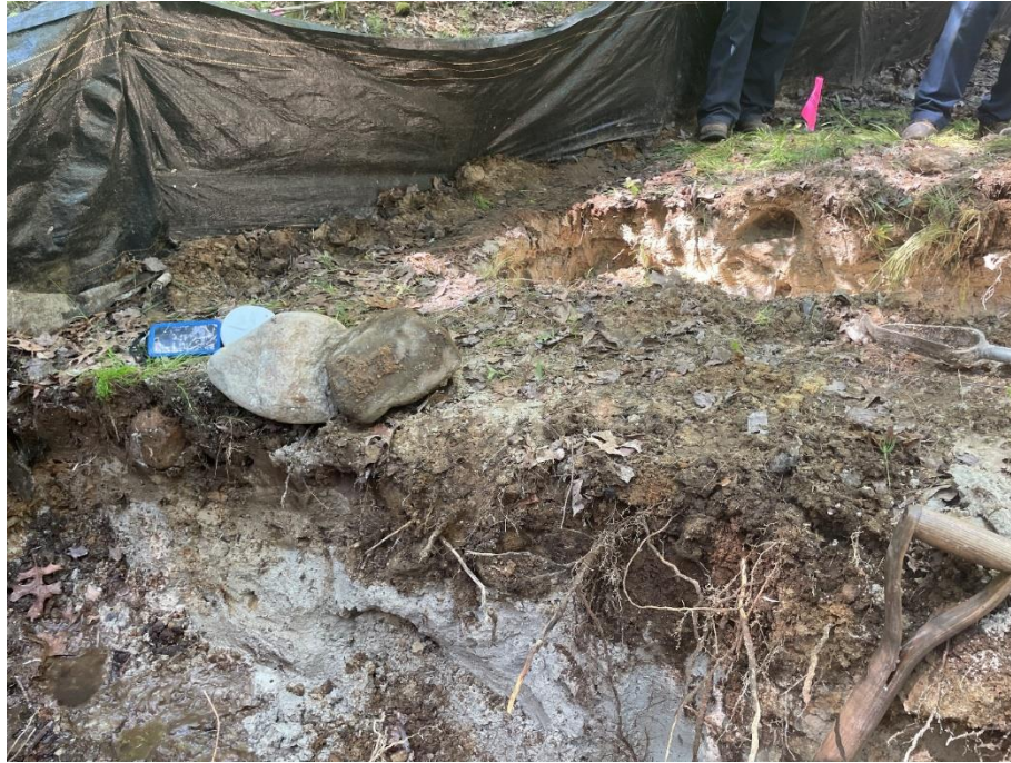
Photo 7 View north of Trench 2 in the forefront and Trench 1 in the background (6/22/23).
