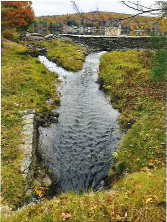
Figure 4: Split stream channel upstream of culvert.
