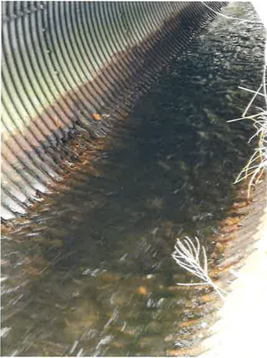
Figure 3. Close-up of corrosion in existing culvert
