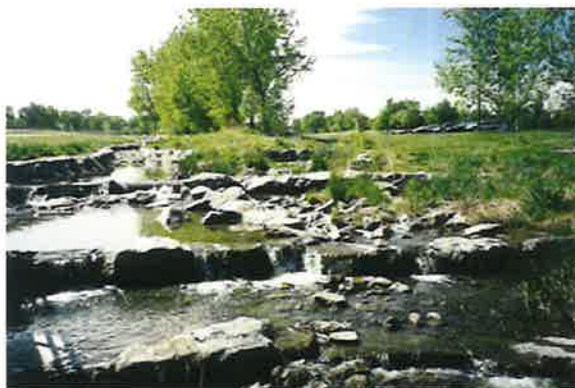
Photograph 9-2. Grouted stepped boulder drop structures such as this one in Denver’s Bible Park can be safe, aesthetically pleasing, and provide improved aquatic habitat besides performing their primary hydraulic function of energy dissipation.
