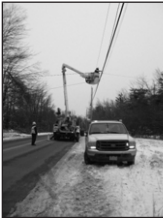
A welcome sight: A utility crew from West Virginia restores power using trucks sent from Indiana.
