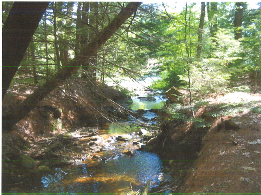
Photo # 6 – Fiske Pond Spillway, Eroded Outlet Channel
