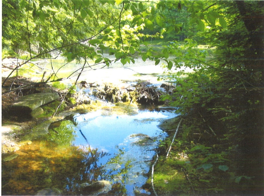
Photo # 5 – Fiske Pond Overflow Spillway, Beaver Debris
