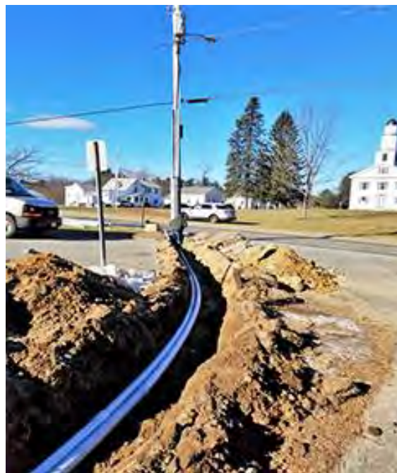
New Conduit Burial from Cooleyville Road to our hut behind Town Hall
